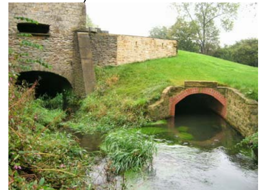
Original mill on left with waterwheel arch. Turbine house on right (new stone work) and outflow tunnel.
